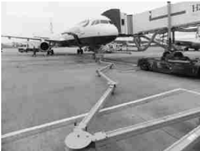
Apron Cable Electricity Supply
